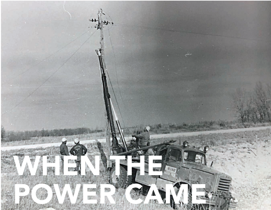
Rosebud Electric Cooperative providing power in the early days. Photo provided by the Rosebud Electric archive.
